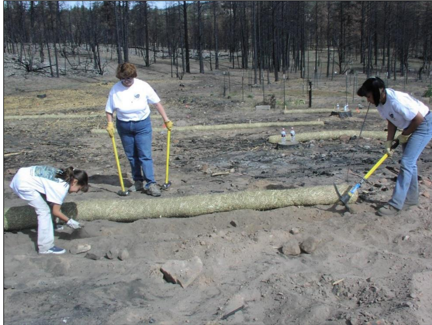
Figure 7-17. Volunteers install fiber rolls (also called wattles) on burned area prior to Critical Area Planting (342) to control erosion. Photo: USDA NRCS.
